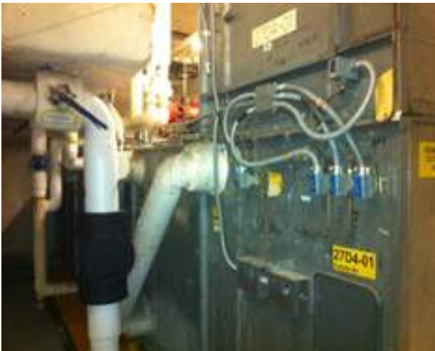
Underperforming central station AHU
