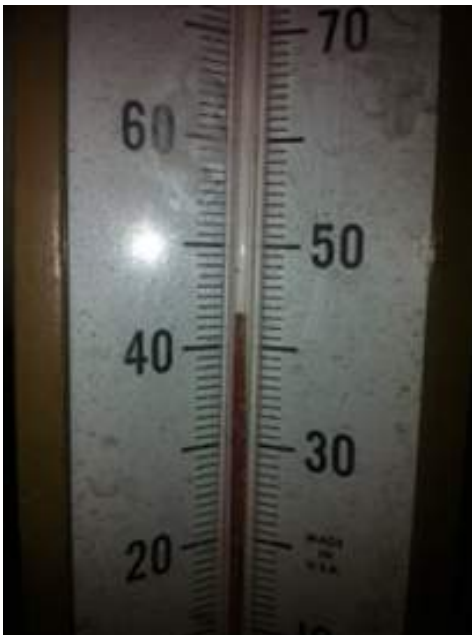
43°F chilled water supply
