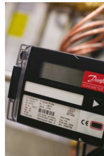
The installed Danfoss substations are all equipped with a heat meter, type Sonometer® 1000 enabling individual billing according to actual consumption. Photo: Anna Kari ©
