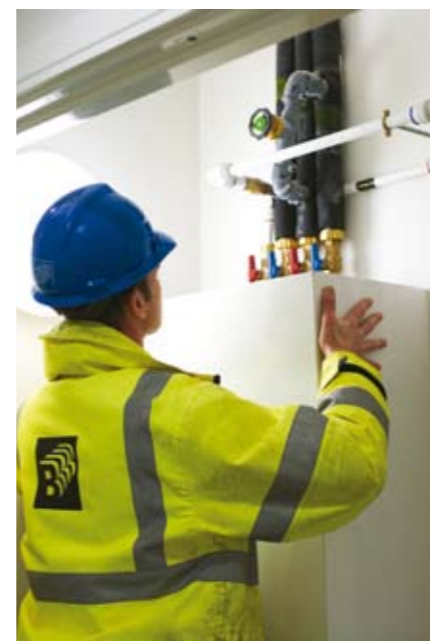
Project engineer Simon Angold from the constructor N.G. Baileys is satisfied with the fact that the new energy effective system at Highbury demands much less space than a traditional boiler. Photo: Anna Kari ©
