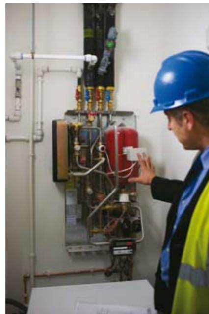
Project manager Ian Stripp from SAV Modules is controlling a Danfoss substation in a flat in the former art deco West stand at Highbury Stadium. Photo: Anna Kari ©
