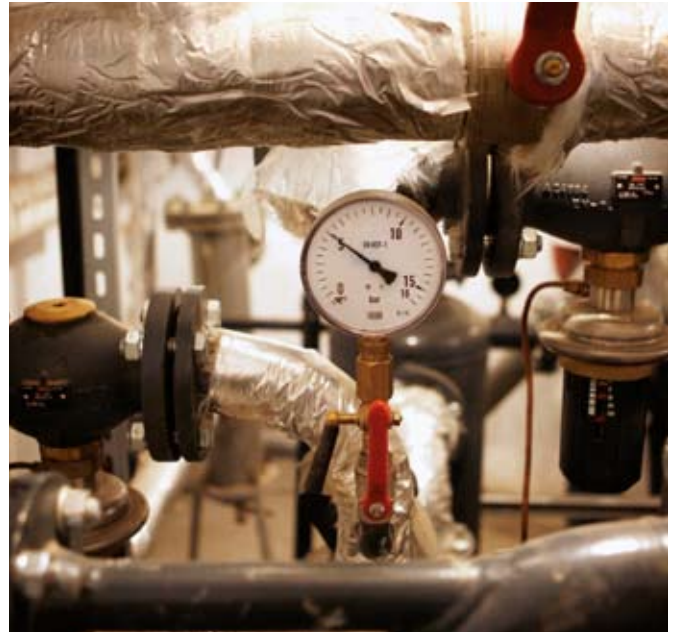
The new substation from Danfoss is squeezed into a 3 times 3 square meter room in the cellar in one of the buildings, but is anyway supplying 220 flats
